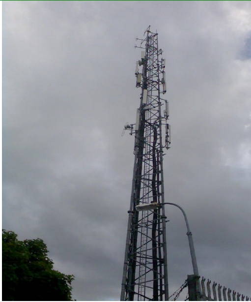
Transmitter Site Photo
